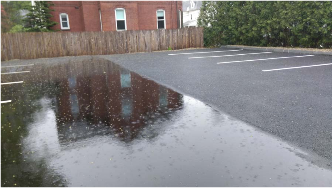
The Mandelle parking lot during a rain event in May. The permeable side (right) completely absorbed all the rain falling during this event. (Photo by Peter Gagnon, Facilities Management)
